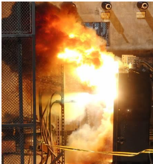
480-V network protector with a live transformer
