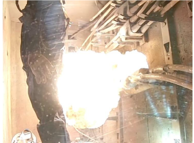
Underground splice failure
