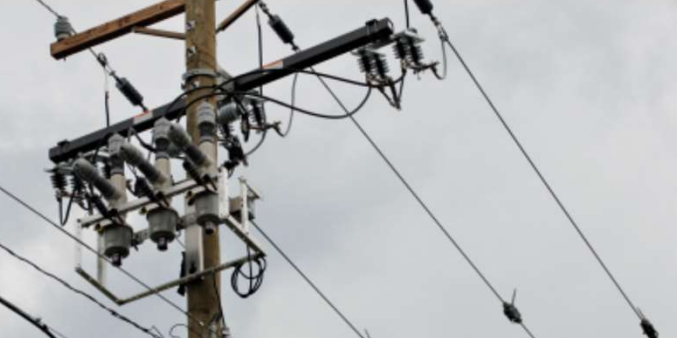
Distribution Automation Assets Research on distribution automation practices, systems, and equipment
